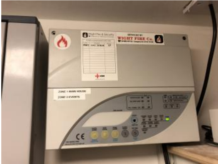
Alarm control panel
